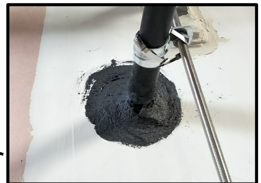
FYREPEX™ Sealant filled to the full depth of the plasterboard on both sides of the wall
